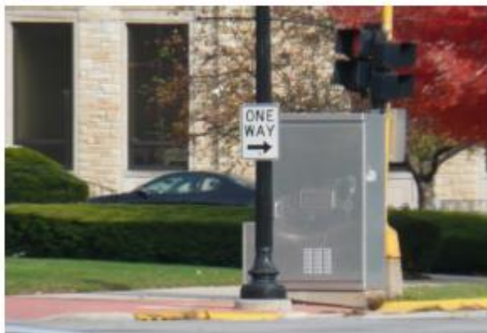
City fiber traffic pedestals we may have access to.
