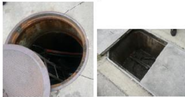
Existing fiber access points.
