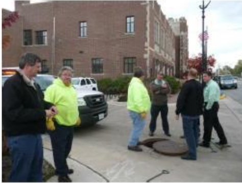
Access to the cities dark fiber and open conduit.
