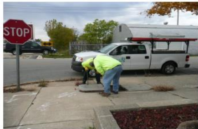
City crews were very helpful opening manholes and checking possible fiber routes.
